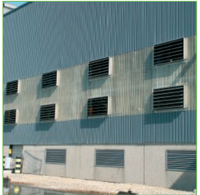
View of the ventilation grates in the facade of the lead refinery. The investment led to a significant reduction in the emissions from the building ▲
