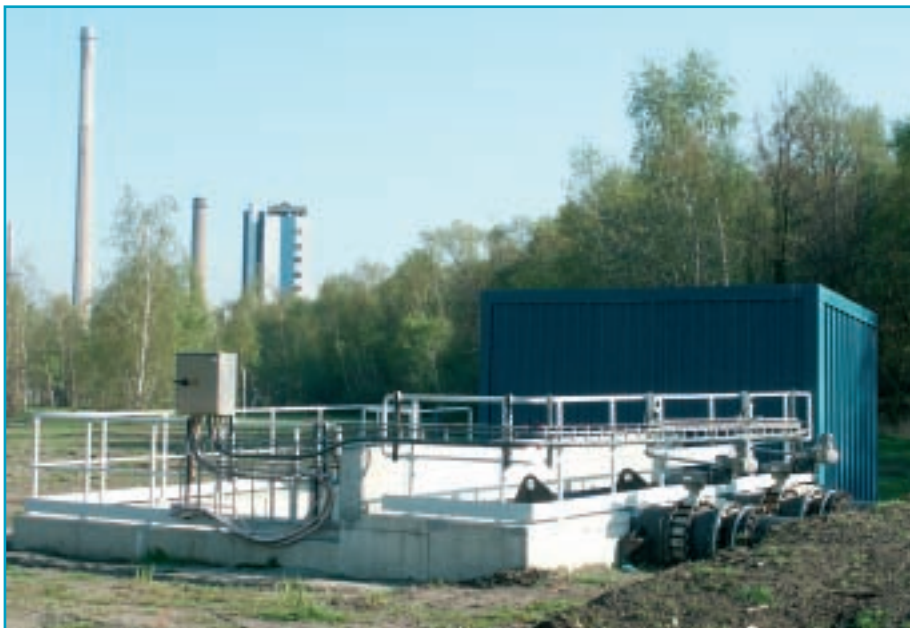
▲ | View of the storm pumps which during intense rainfall can divert peak flows up to 7,000,000 l/h to the water treatment plant.
